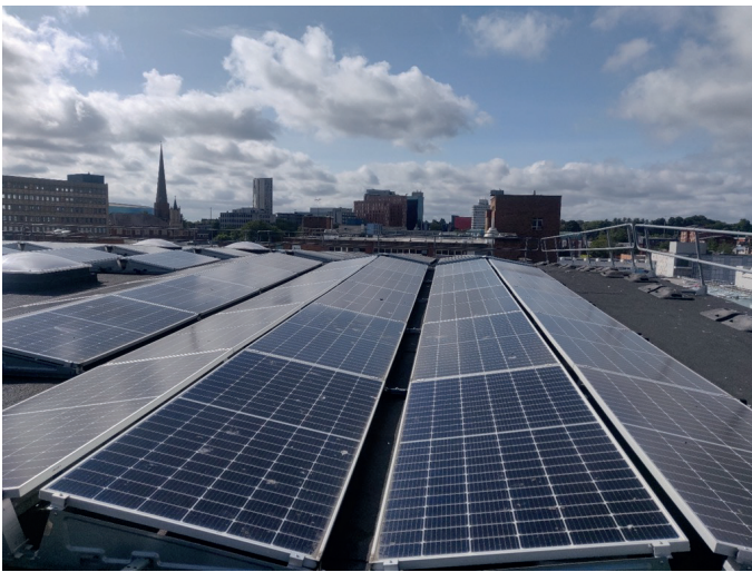
Figure 14 – Solar panels on the roof of Central Library
